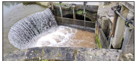
Back in action, feeding water through to the canal, not the river.
