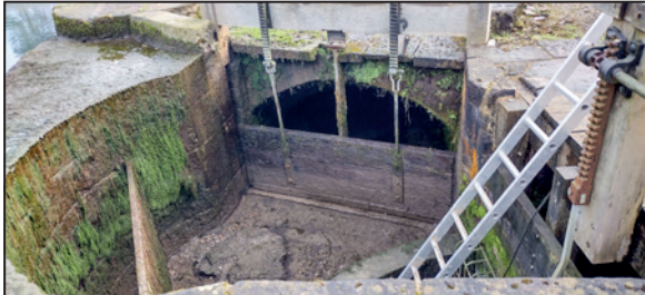
The leaking sluice paddle with twin lifting racks which should only allow water to pass when the level reaches the top. The protective trash screen has been removed and stands on the left. The feed to the canal is through the grill on the right.
