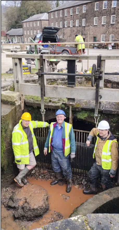
Job done! Trash screen replaced and ballast over the bottom of the rubber skirt. (l to r) John Britten, Les Hall and Ian Hutchinson, with John Guylar behind the camera and John Boucher reloading his trailer.
