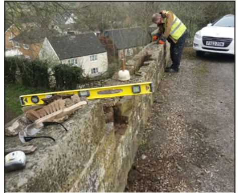
Laying out the damaged wall at Sawmills to lay the new stones.
